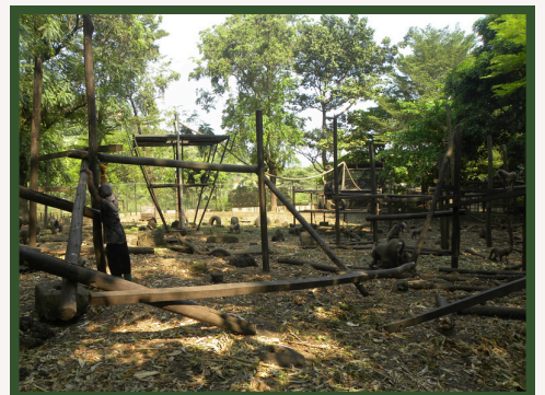
Making repairs to our drill climbing structures, which often are broken by the adult male drills displaying their strength to the rest of the group.
