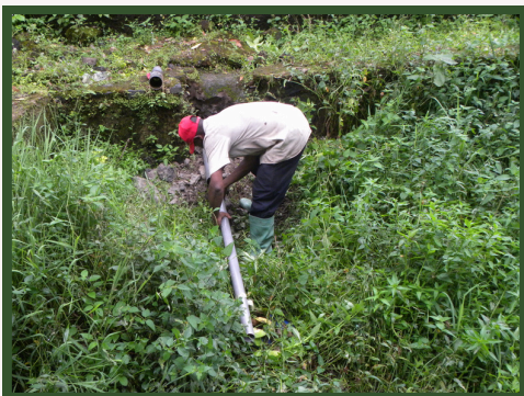
Repairing the pipe that drains the chimpanzee island pool to ensure it is fully functional for the dry season. Watch Eve enjoying the pool here!
