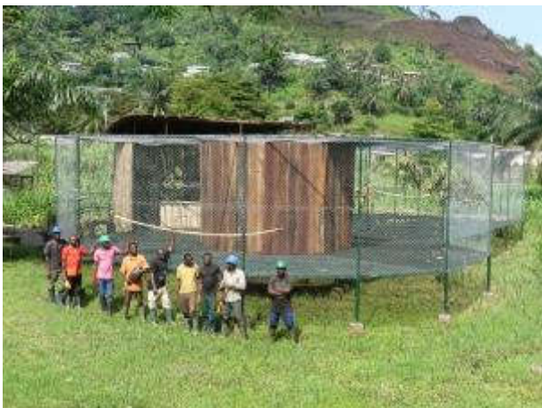
Image 5. Our construction team builds and maintains all our infrastructures. Here, the large aviary.
